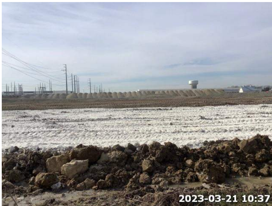
Photo 4. View of grading activities from northern edge of the Project area. Photograph taken facing south.
