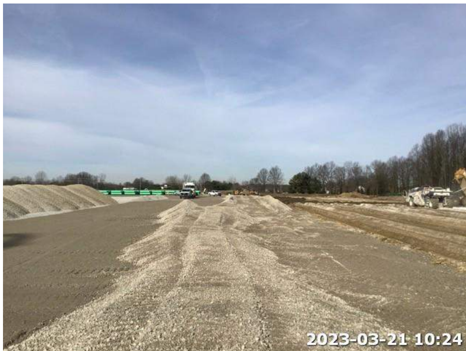
Photo 6. View of grading activities in southeast corner of Project area. Photograph taken facing west.
